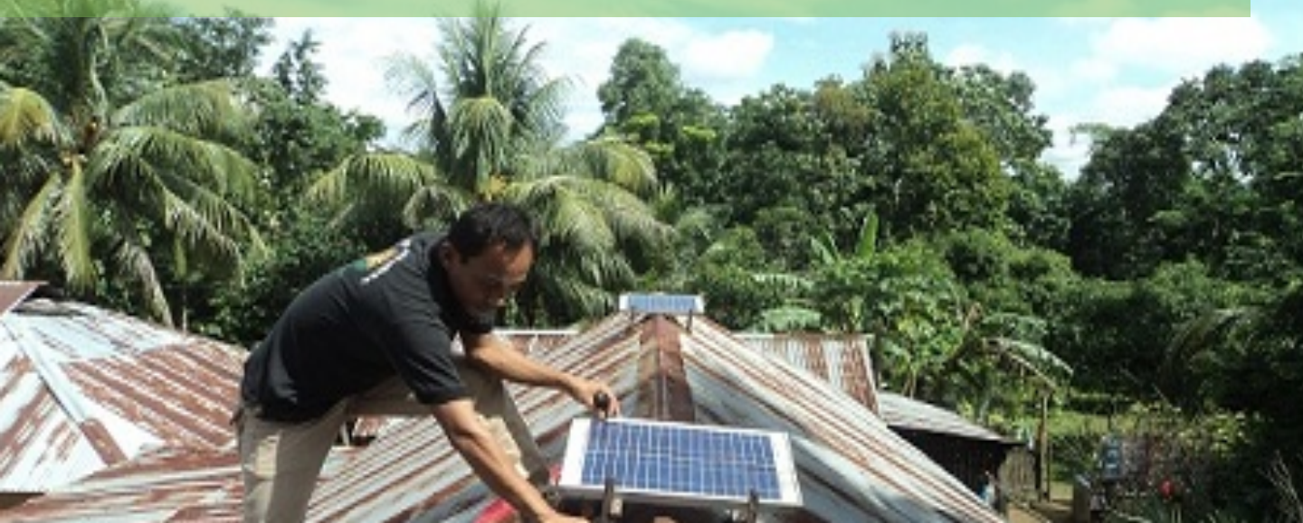
Solar Home System Installation in a rural area of Bangladesh by Bright Green Energy Foundation
